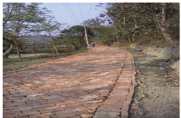
Brick soling from Krishnarai Para to Pohor School at North Longtharai V.C (NREGA)
